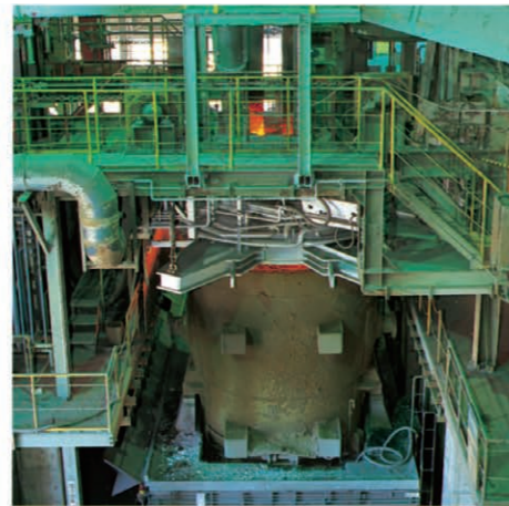
炉外精錬設備 Ladle-Refining Process Equipment
