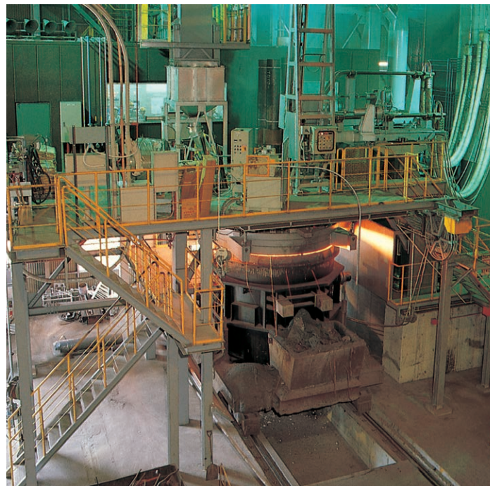
取鋼精錬 Ladle refining
